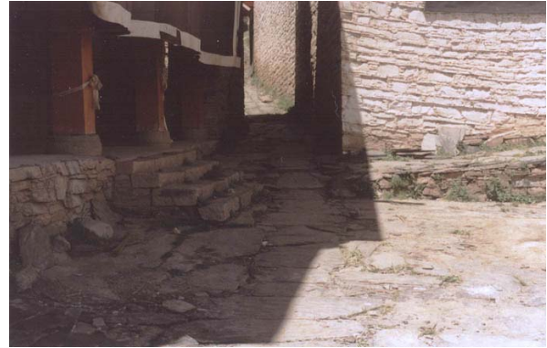
Drainage running in front of the Protector Temple consists of a trench covered with slate. While this does lead water away from the east side of the building, it does not catch the water running into the north wall.
