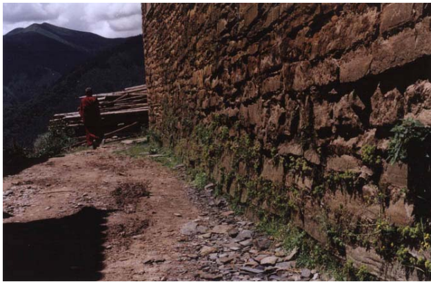
South exterior wall of the Protector Temple with extensive plant growth at the base, evidence of excess moisture in the building fabric. The roof of the nearby kitchen (note shadow) and the roof of the Protector Temple shed large amounts of water into this narrow alley during downpours. Lack of adequate drainage results in moisture creeping up the walls of the building through capillary rise.
