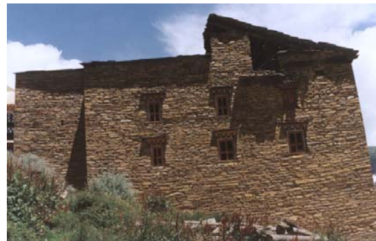
Exterior west façade of Protector Temple with replacement windows that are paneless and unglazed. The lean of the south wall is visible from this perspective.
